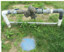
Irrigation manifold for landscape irrigation at Airforce Base in Dayton - OH
