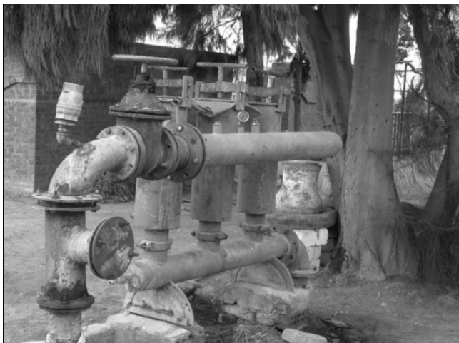
FIGURE 7.7 Pumping and filtration units for drip irrigation system.
