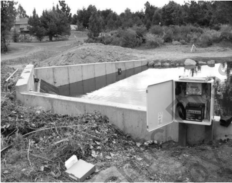
FIGURE 9 Measurement of water flow in an irrigation ditch, using the Stevens AxSys Flowmeter [12].
