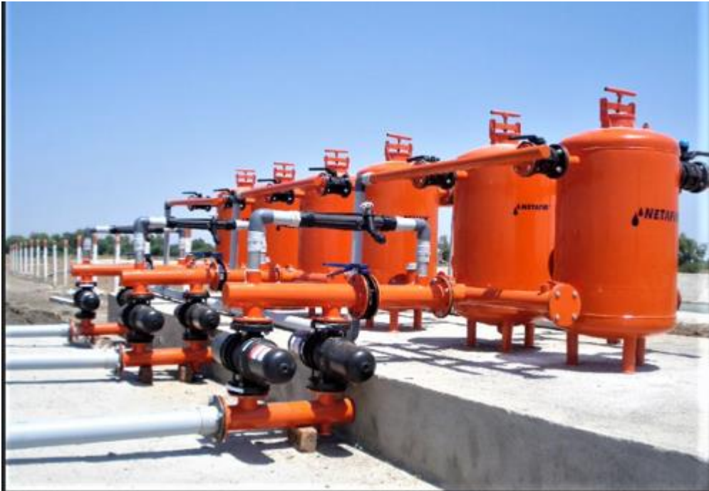
Sand Filter Battery
